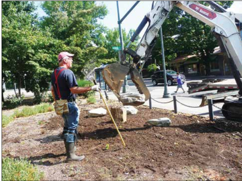
John Barker of the Hardy Plant Society watches Will Pottratz, of Will & Sons Excavation, guide his machinery to drop a landscaping stone at the Gladys McCoy Memorial Garden. Volunteers are continuing to care for the plantings gradually added to the curved garden. (Janet Goetze)
