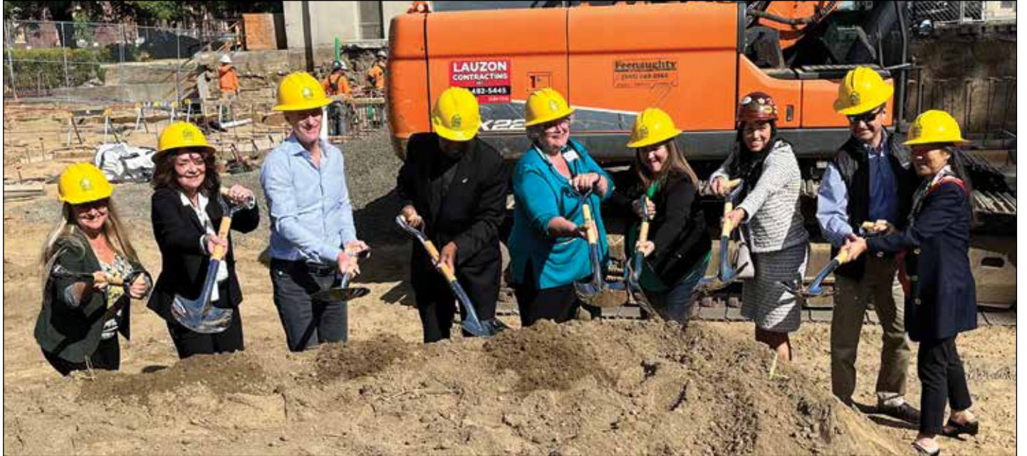
Portland Mayor Ted Wheeler and Commissioner Carmen Rubio were joined by other principals in the mid-September groundbreaking for Francis & Clare Place at St. Francis Catholic Church in Buckman. The Catholic Charities development will add 61 affordable apartments to Buckman. (Phill Colombo)
