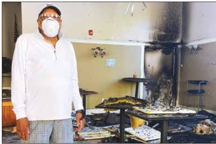
Louis McLemore, leader of the Billy Webb Elks Lodge, surveys damage from a September fire to the building, which has been named to the National Register of Historic Places. (Billy Webb Elks Lodge)
