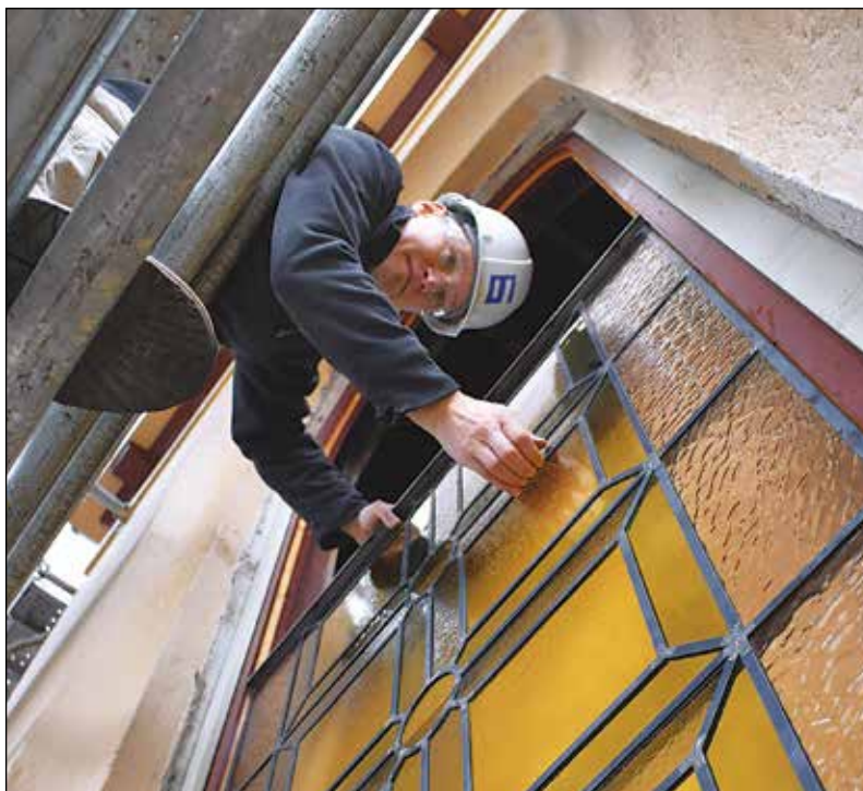
A portion of the St. Rose window is removed for repairs at St. Rose of Lima Catholic Church. Some of the stained glass at the church, dedicated in 1925, was on the verge of falling apart. The repaired window was expected to return before December. (Courtesy of St. Rose Parish)
