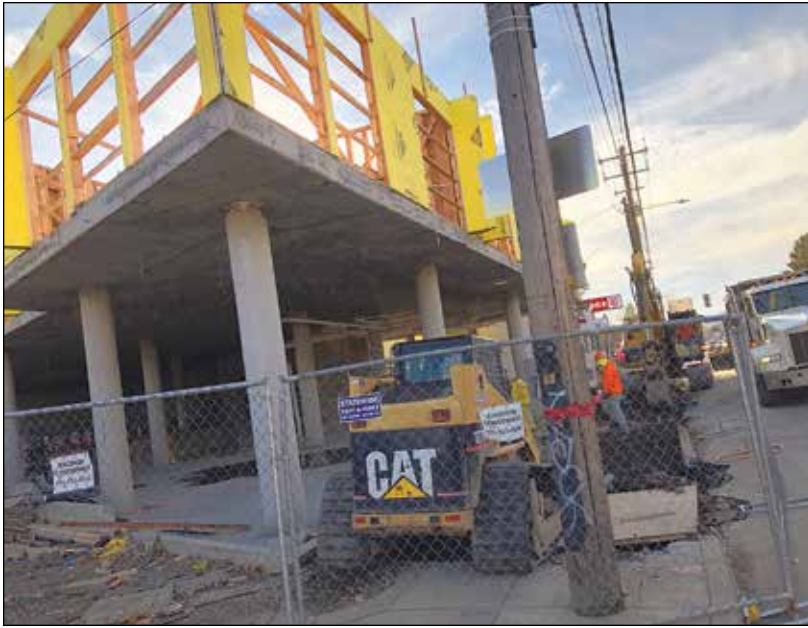
Second-floor framing is complete on the Sandy 51 project at the corner of Northeast Sandy Boulevard and 51st Avenue. The six-story, 85-unit mixed use building, which will have retail space on the ground floor along with a lobby and parking, is being built on the site of the former TacoTime Restaurant. (Phill Colombo)
