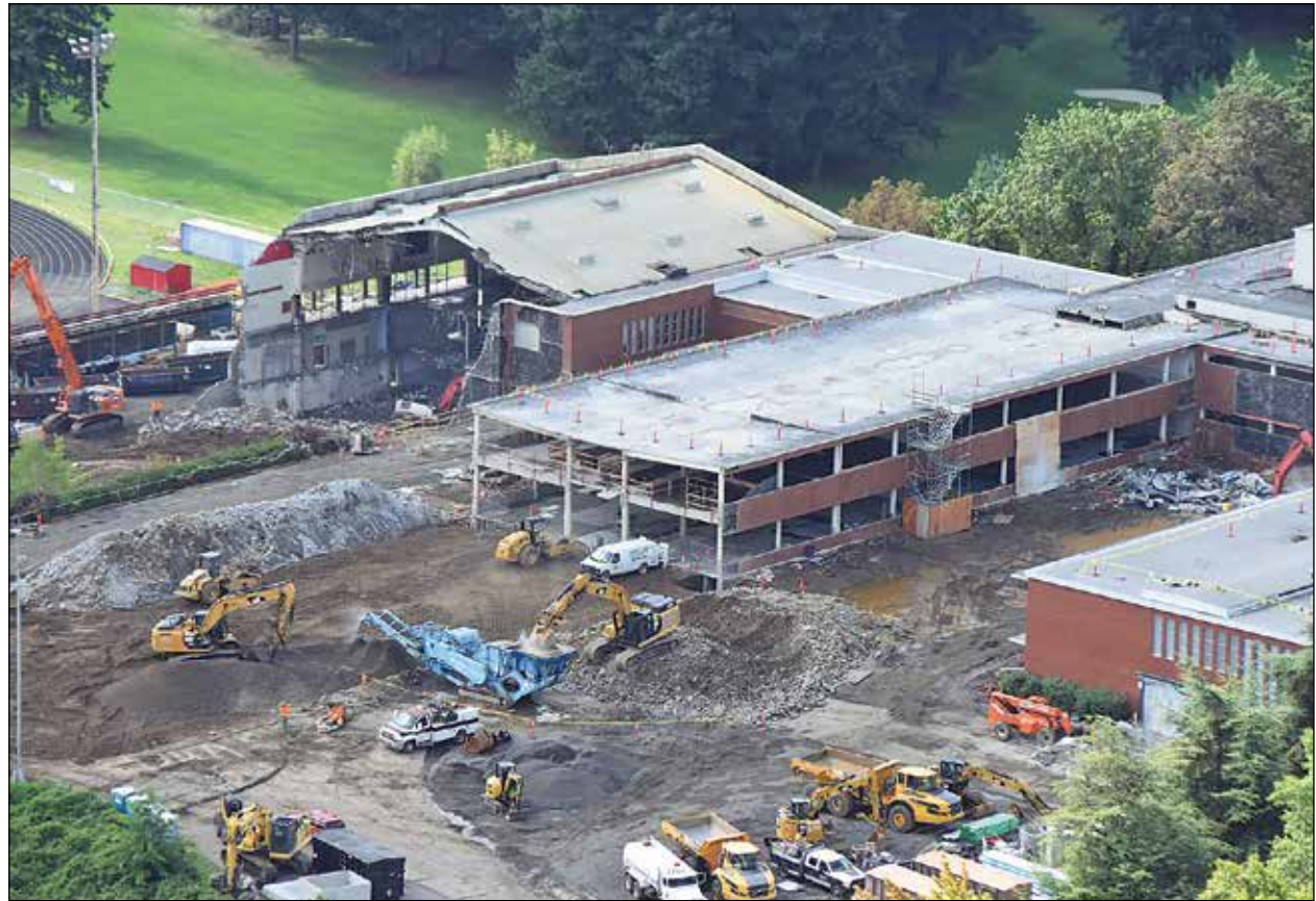
Demolition work has begun on the Madison High School modernization project. (Portland Public Schools)
