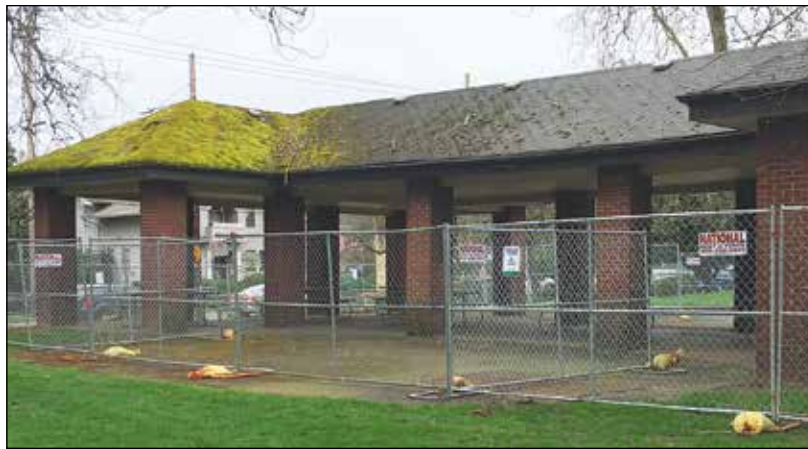
Portland Parks and Recreation has fenced off Montavilla Park's picnic structure. It will be demolished along with a park wading pool. (Portland Parks and Recreation)
