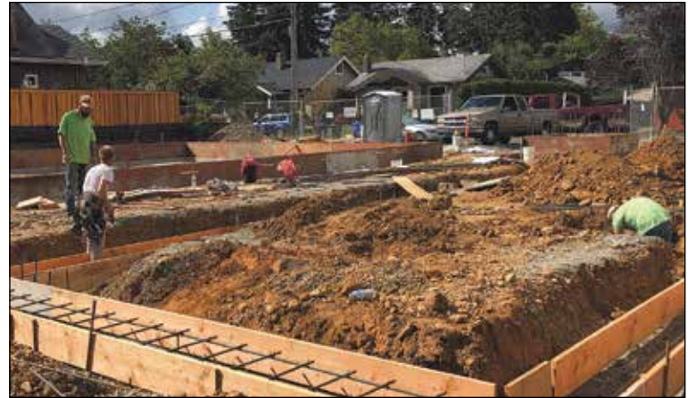
Carpenters and iron workers build forms for the fittings of one building while concrete for a second building dries at the corner of Northeast 51st Avenue and Fremont Street. Grove Development of Beaverton began work on the site of a former Christmas tree lot in late August. (Phill Colombo)
