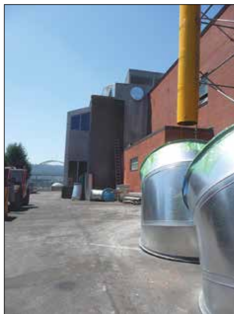
Upgrading is continuing at Tubman Middle School, including a system to remove interior pollutants from Interstate-5 traffic down a hill from the school. However, an air quality report recommends that outside activities be limited, especially during high traffic hours. (Janet Goetze)
