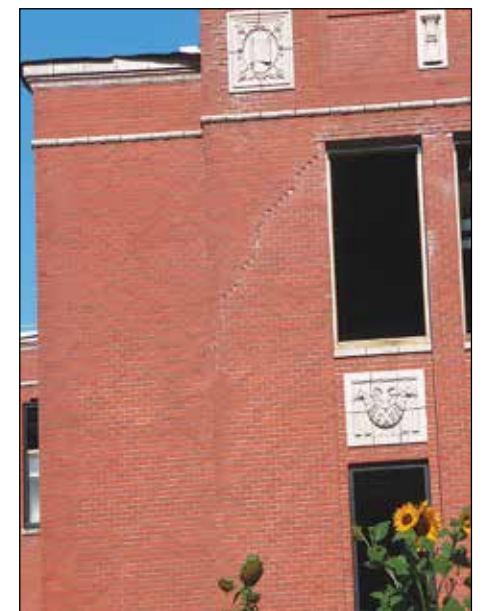
A jagged scar remains in the brick of Grant's north wing, showing damage from rain, heating and cooling that can stress bricks after 90 years. Bricks are being checked for damage and grout replaced in the school's original building. (Janet Goetze)
