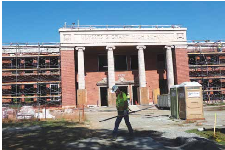
Modernization is continuing for another year at Grant High School where exterior bricks are being cleaned and grouted. The interior, completely gutted, will have new electrical and plumbing systems and newly designed learning centers. Seismic work is being completed. Also planned are a new athletic wing and library. (Janet Goetze)
