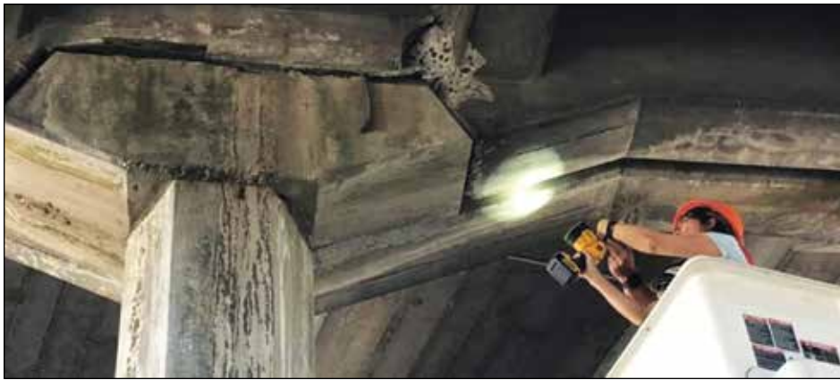
The NE 33rd Avenue Bridge over Northeast Lombard Street is currently closed after engineers with the Portland Bureau of Transportation observed damage to the concrete in one of the bridge's cross beams. (Portland Bureau of Transportation)
