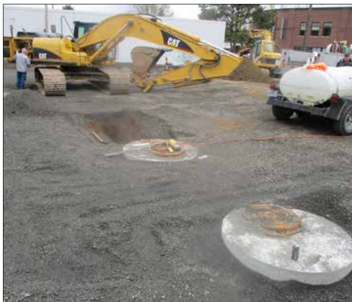
Leveling the property and excavation for sewer and footings began in April on the Sandy 51 project in Rose City Park. A six-story, 85-unit, mixed-use building will replace the former TacoTime Restaurant at 2351 N.E. 51st Ave.
