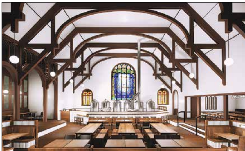
Work on transforming a church at 2400 N.E. Broadway into the Steeplejack Brewing Co. is expected to be completed this summer. Partners Dustin Harder and Brody Day are planning a celebration to welcome neighbors to their new space. (Steeplejack Brewing Co.)
