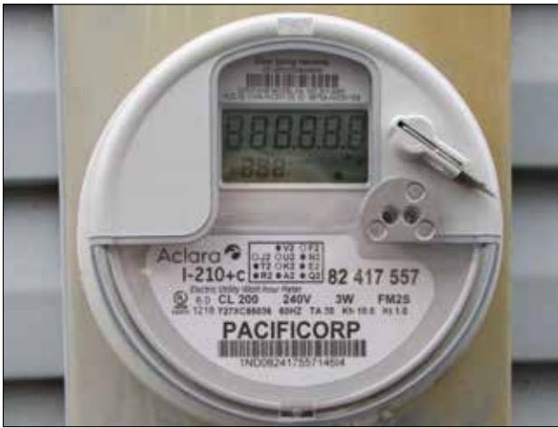
One of the 20,000 new digital smart electricity meter installed by Pacific Power over the past month. Part of a $117-million investment, the meters will give customers more knowledge of how they use electric power and how they can make changes to save. (Phill Colombo)
