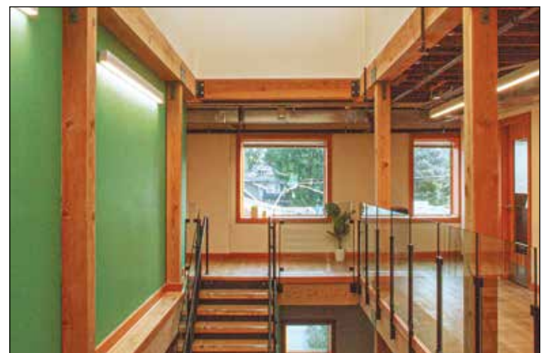
A new skylight on the Rothert Building's third floor allows enhanced daylighting in the building's core, flooding a stairway and common areas with natural light. Built in 1922, renovation of the Hollywood district building is scheduled for completion by its 100-year anniversary. (MCA Architects)
