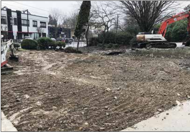
The former Tonic Restaurant in Kerns is no more. In January, the city issued a demolition permit for the structure, built in 1929, to make way for a new five-story, assisted living facility with 65 off-street parking spaces. (Phill Colombo)
