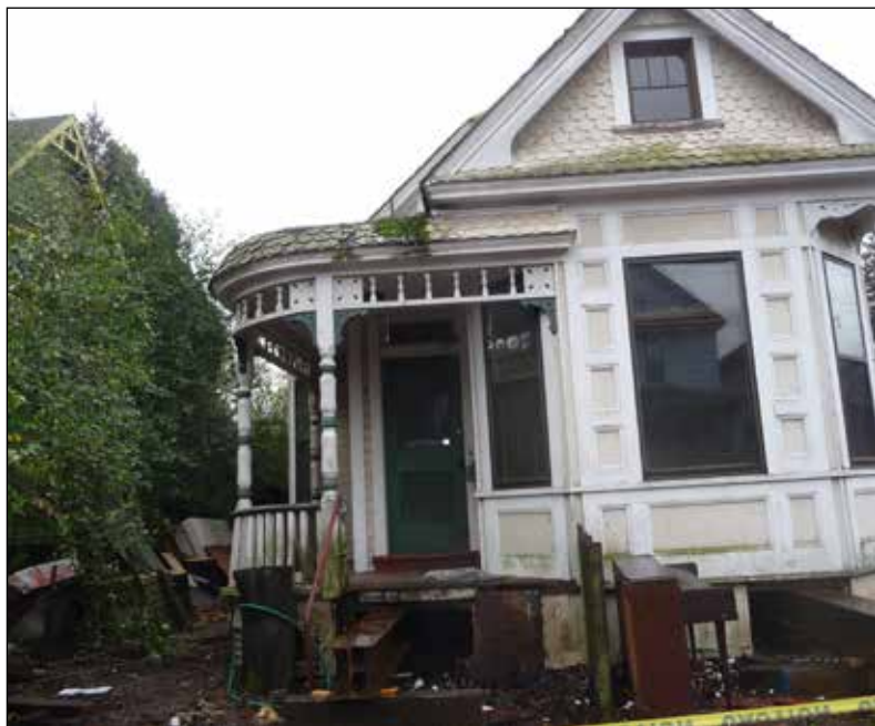
The Queen Anne-style Mayo house, built in 1895, is jacked up for a move on Northeast Sacramento Street to Davis family property. A city decision prevented the family from rehabilitating a building on the land in 1982. Now the Davises can rehab a building to include art and history of the African American diaspora from the Eliot neighborhood. (Janet Goetze)
