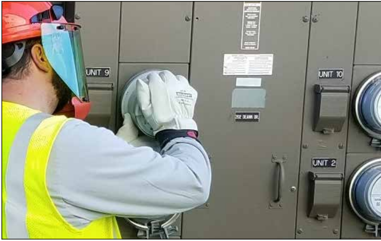
An Aclara installation team updates a Pacific Power electric meter, giving almost 80,000 Portland homes and businesses access to informative and useful power consumption data. Pacific Power said the new meters will also enable the utility to cut power costs. (Pacific Power)
