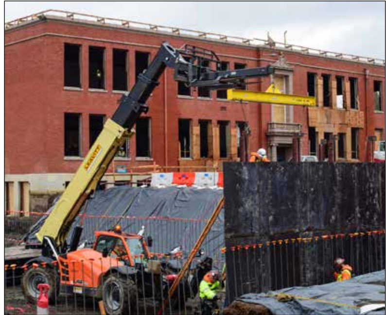
As the Grant High modernization project moves forward, the original entry to a 1923 structure known as the 'old gym' is visible for the first time in six decades. Students are slated to return to campus in the fall of 2019. (All photos by John Butenschoen)
