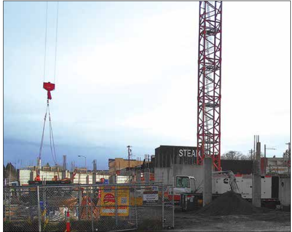
Construction of the first floor of a new six-story building at 2069 N.E. Sandy Blvd. begins to show structure above ground. The building will house basement parking, ground floor retail and 206 studio, one- and two-bedroom apartments.
