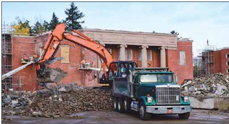
Demolition and construction work continues on the project to modernize Grant High School. (John Butenschoen)
